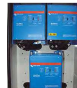
Battery inverters / chargers
