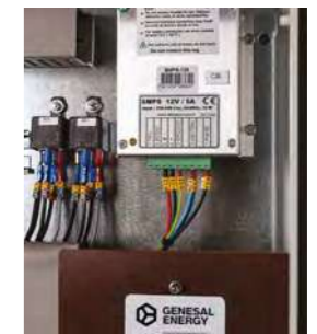
Engine battery maintainer from external grid
