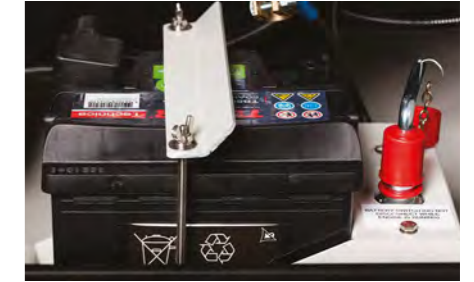
Battery with battery switch
